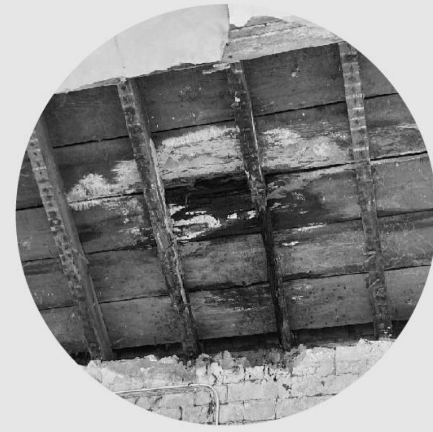
Damaged wooden structure
