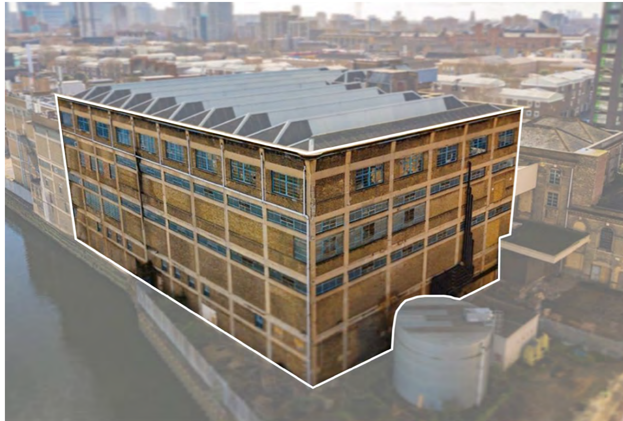
Exterior elevation made up of London stock brick infill walls looks almost modular with the RCC framing structure. Weathering effects due to rain and heat are seen along the facade creating a palette of ochre hues.
